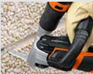
Dust extraction is used when working with hazardous grout materials (e.g. PCB).
